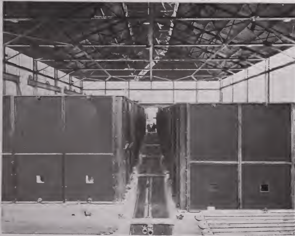
LOOKING DOWN CENTER OF HEAT TREAT OVENS
